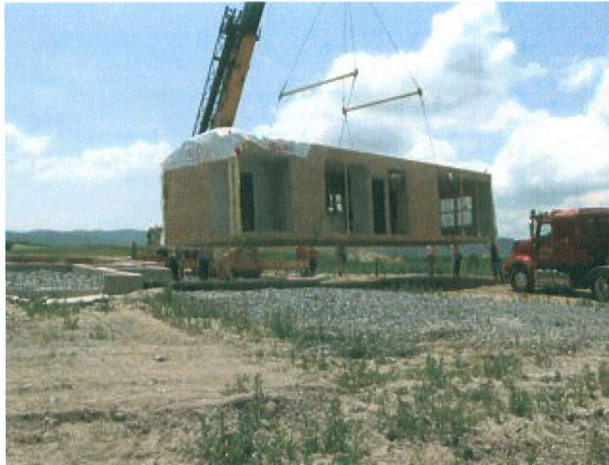
Modular housing is vulnerable to the North Country elements upon arrival. Here, a piece of one of the Lewis Family Farm employee cottages is craned into place.
